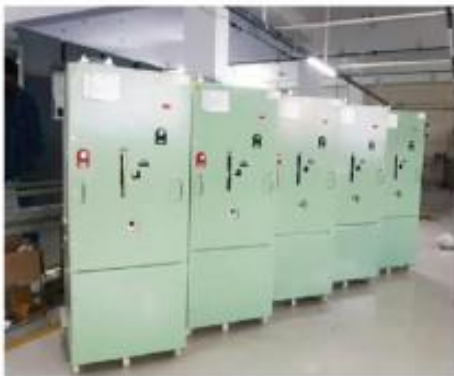
VCB 6.6kV MLIP Cluster projects
