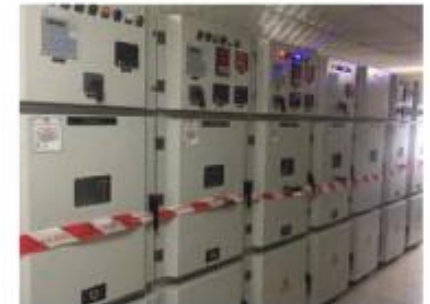
T&C of 11KV Switchgear for M/s. Petrosa Global
